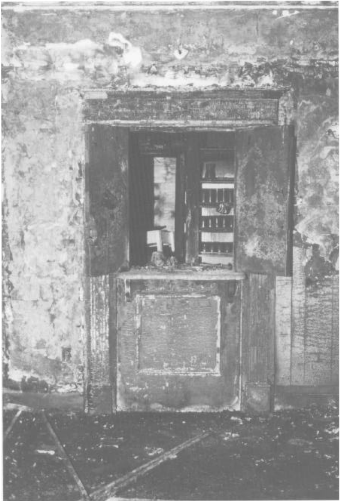
This view of the dutch-style service door to the bar room shows the deep charring to the door frame above the opening and the plywood paneling on the lower right side of the door opening.
