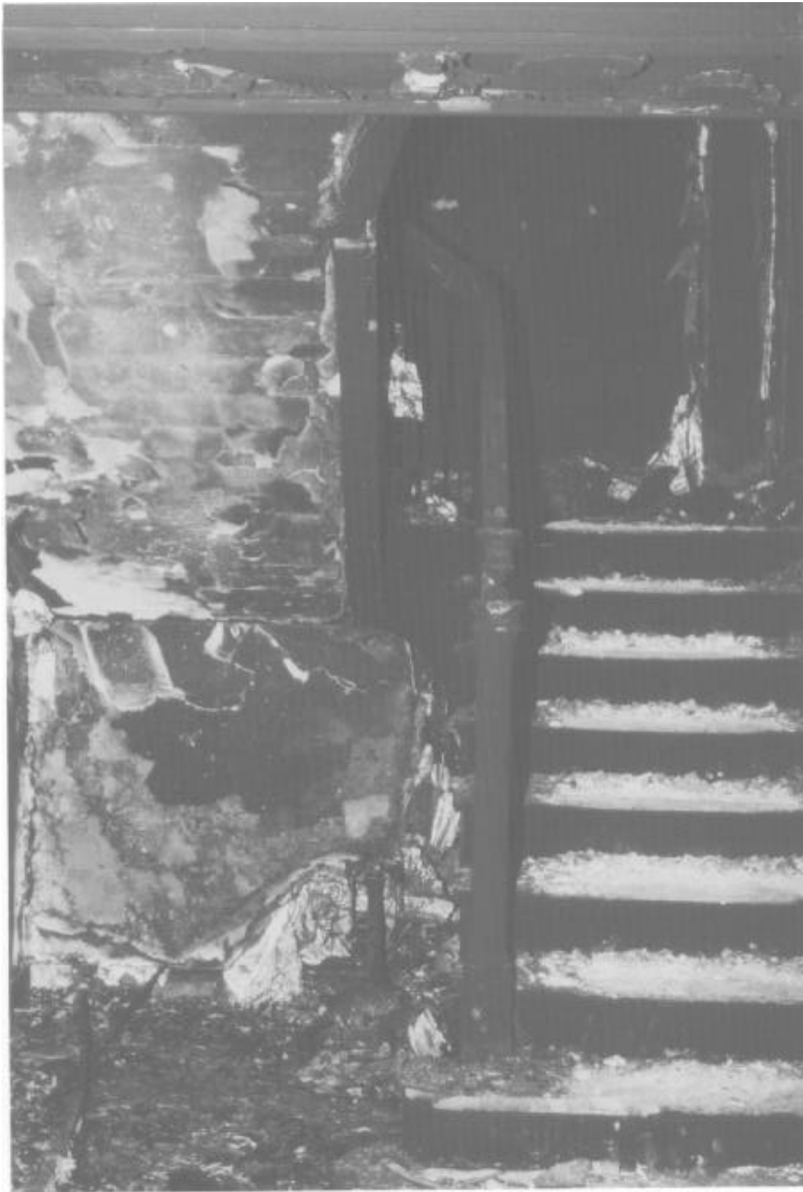
View of east stairway connecting third through ninth floors. This stairway was open on the third floor (shown here) and the fourth floor permitting the stairway to fill with smoke and the fire to spread vertically to the fourth floor.
