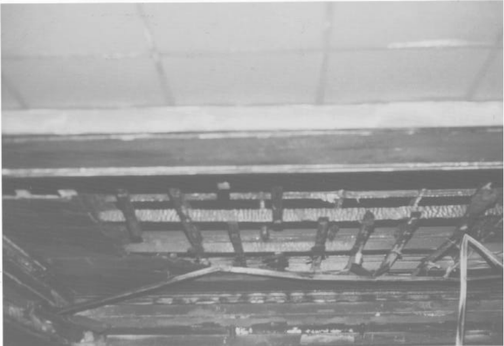
View of suspended ceiling damage above the location in the grill room where Captain Spalding was found unconscious and covered in debris.
