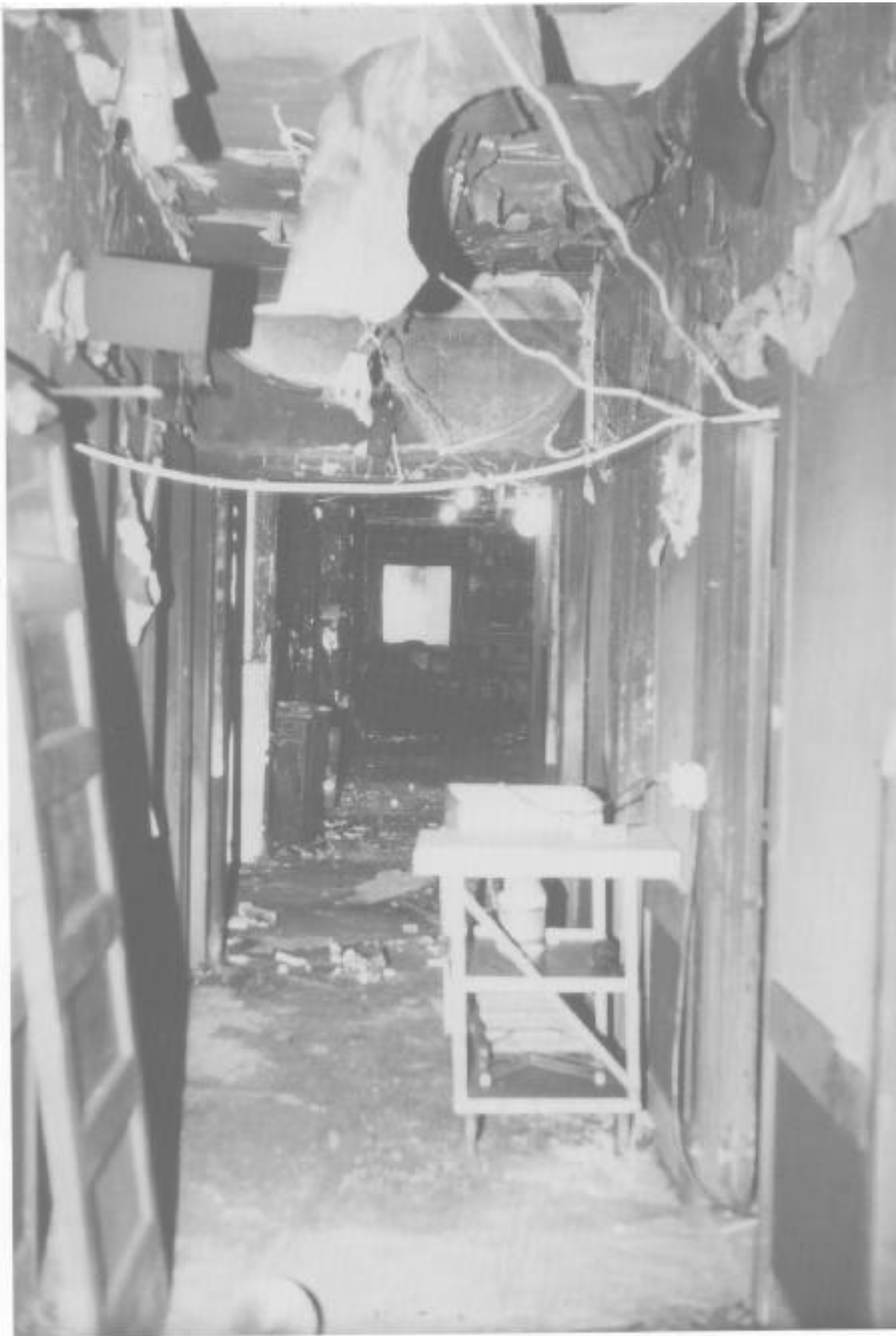
View of third floor service corridor looking east from standpipe cabinet. Note the relatively minor damage. Most of the damage is confined to wall and ceiling finish materials.
