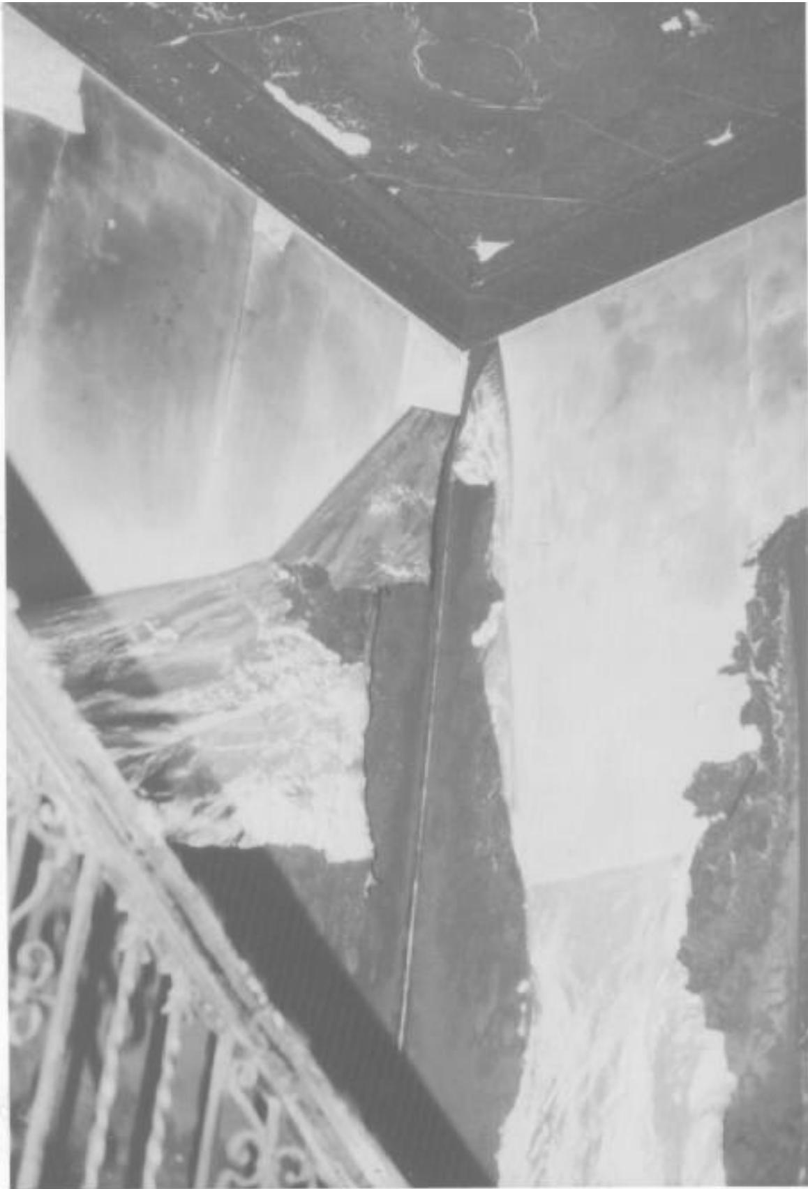
This view from the monumental stairway looking up toward third floor ceiling shows relatively light damage to the cornice, but heavy damage to the combustible foil-backed wallcovering.
