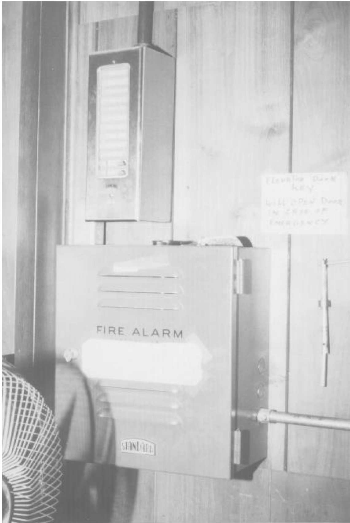
Manual fire alarm system cabinet and tabular fire alarm annunciator above. This system provided power to the fire alarm signals on all floors.
