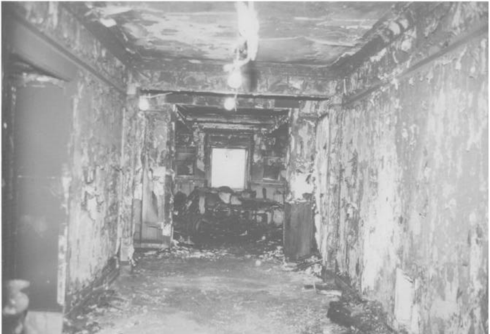
This view of the third floor corridor looking east toward the large dining room shows the extensive damage to combustible wallcoverings.
