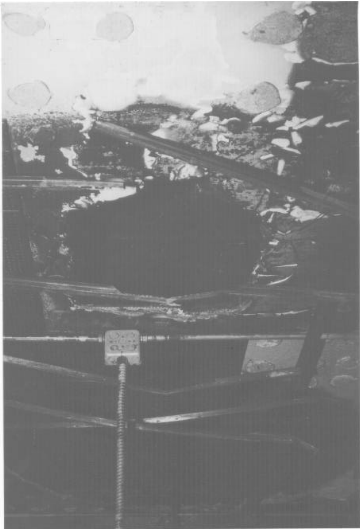
View of opening in suspended ceiling in the McHale Room. Note the charred 1-foot ceiling tiles (at left) glued to the underside of the plaster suspended ceiling and the remnants of the aluminum suspended ceiling frame.
