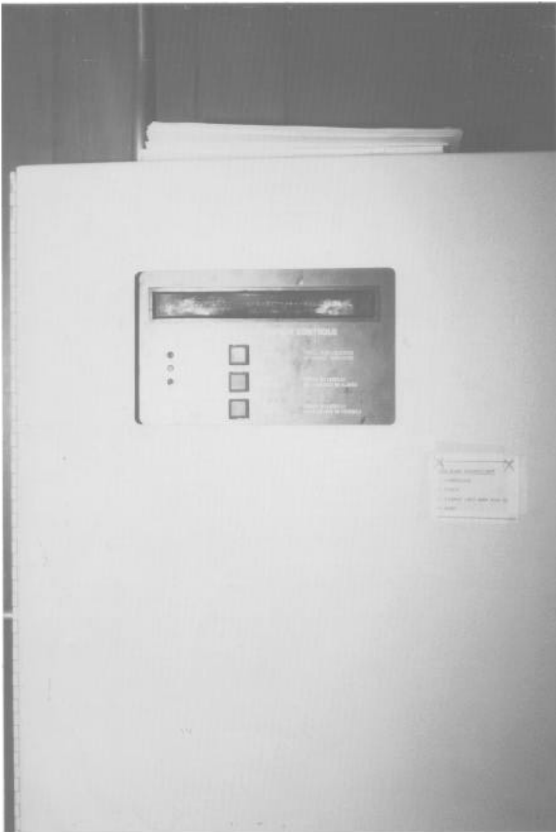
Analog addressable smoke detector control unit. This unit powered and supervised the in-room and basement smoke detectors as well as monitoring the conventional zoned control units which powered the corridor smoke detectors.
