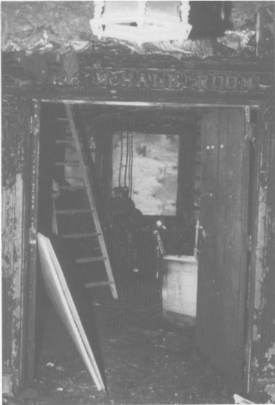
Entrance to the McHale Room looking north from the elevator lobby. Note the fire damage to the wall coverings above the door and the relatively light charring of the door frame.
