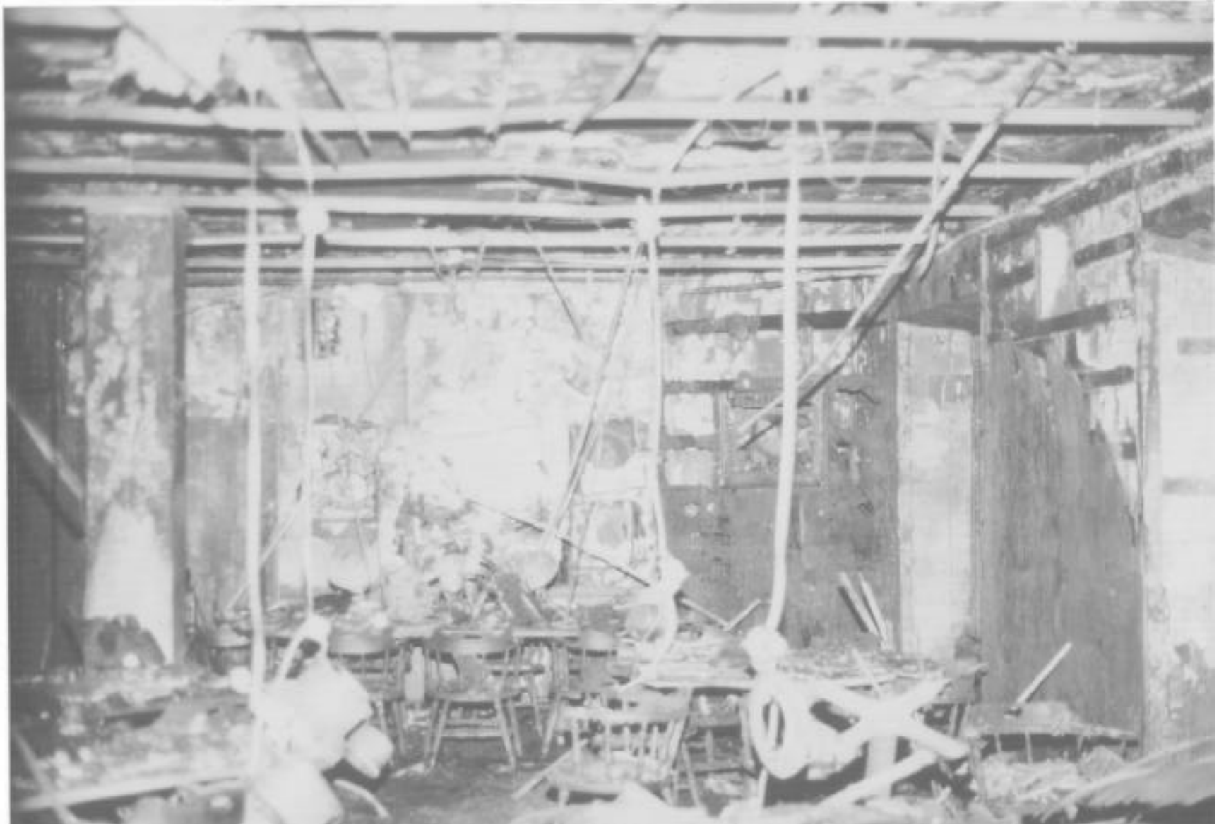
The inside of the McHale Room looking west. Shows the use of furring strips under the wall paneling. Much of the paneling at the remote west end of the room remains intact. Also note that the tops of the chair backs are only slightly blistered.
